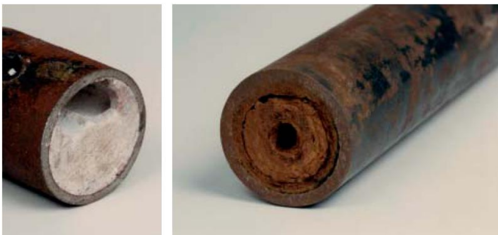
Boiler scale on water side
